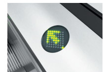
LED traffic lights located in the decking
